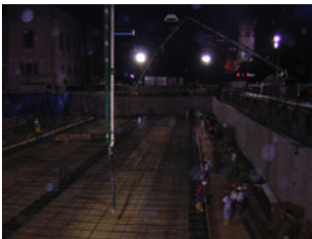
Night has come and the pouring for the first slab-on-deck has begun
