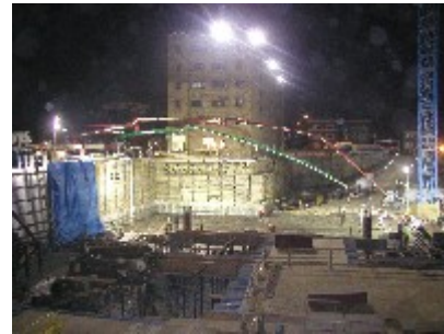
Concrete pumping trucks with extension arms are positioned on Ninth Street overlooking the work site
